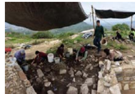
THE EXCAVATION TEAM (BRANDON AGOSTO IN THE CENTER) EXCAVATING PORTIONS OF A RESIDENTIAL PALACE WALL
